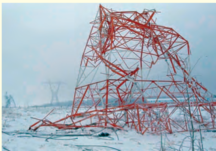
Failed tower due to the severe 1998 ice storm in Canada
