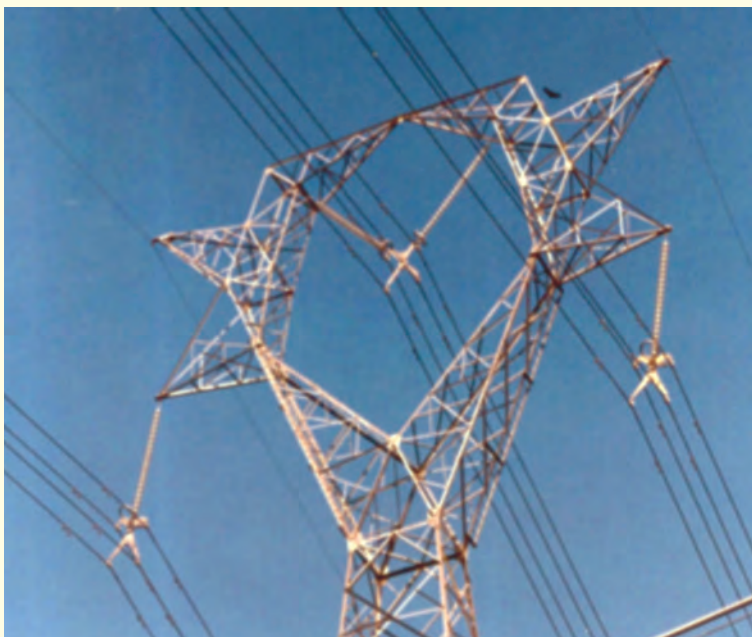
Expanded bundle in a HSIL test line in Brazil
