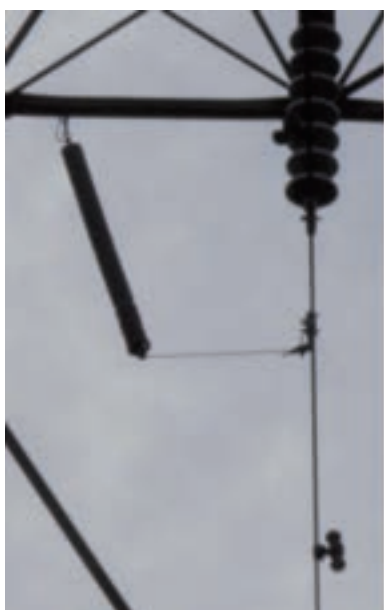
Flexible disconnect lead and arrester as originally installed
