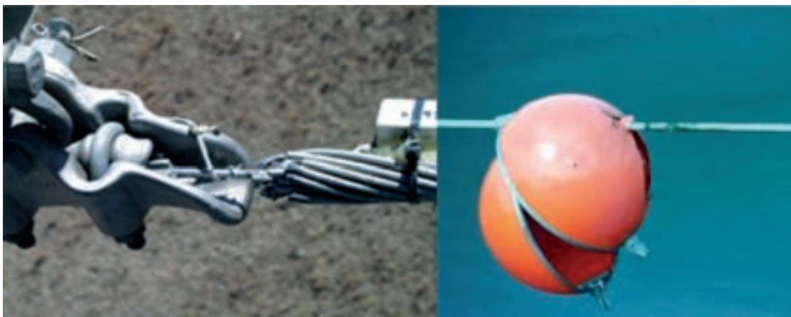
Fatigue failure at suspension clamp
