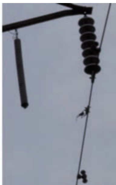
Flexible disconnect lead failed after seven years in service
